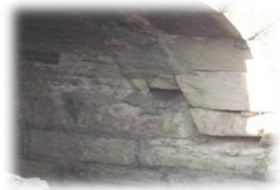
Figure 17. Stone disintegration for opening No. (4)
