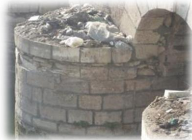
Figure 16. Loss of some mortar parts for stones and disintegration of some of them for opening No. (3)
