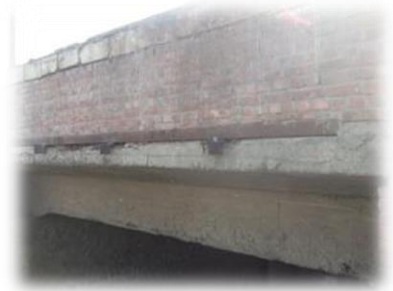
Figure 5. Poor state of façade and loss of some wall bricks
