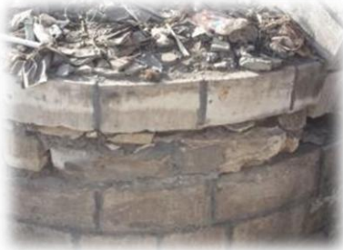
Figure 15. Loss of some mortar parts for stones and disintegration of some of them for opening No. (2)
