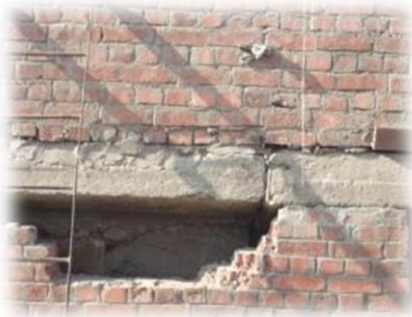
Figure 3. Fall of the concrete cover of the barrage slab
