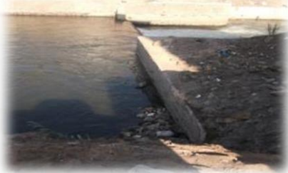
Figure 7. Accumulation of amounts of debris into the waterway
