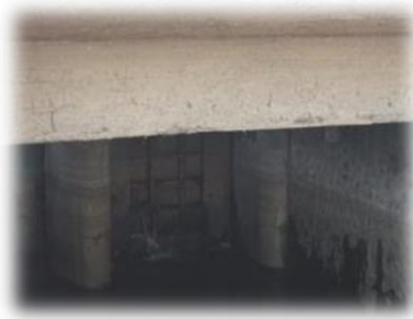
Figure 4. Loss of the concrete cover from slabs and beams of the barrage lock bridge
