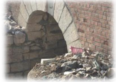
Figure 14. Loss of some mortar parts for stones and disintegration of some of them for opening No. (2)
