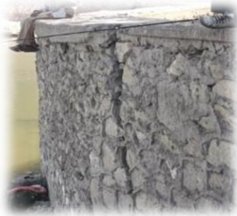
Figure 12. Crack occurs in the lateral stone wall supporter
